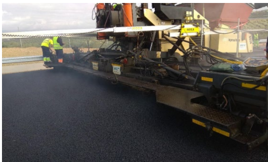
Extension of the wearing course layer in the regulatory exception section on the A-32 Villacarrillo-Villanueva del Arzobispo.
