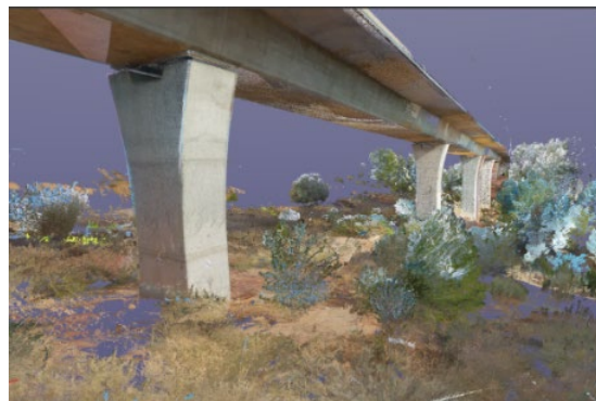
Development of a first “point cloud” of the viaduct for the ERJU project
