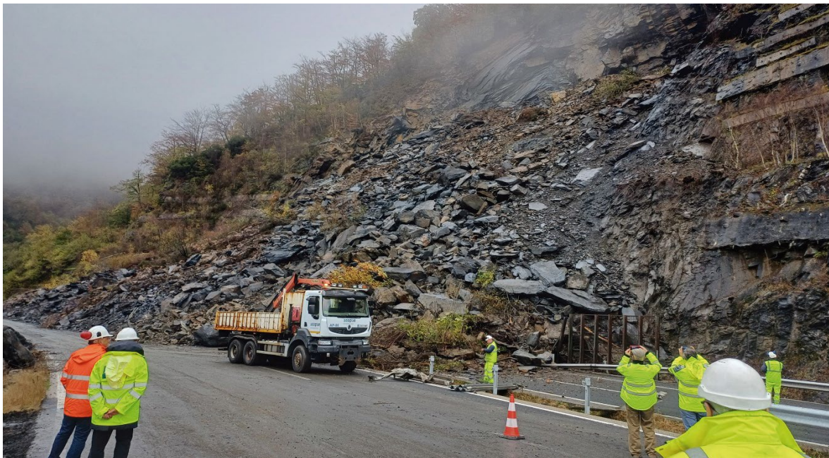
Rockfall on the AP-66 motorway
