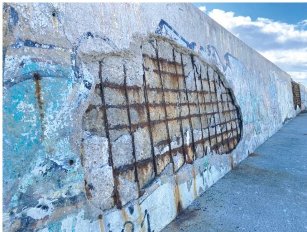
Typical damage to coastal structures.
