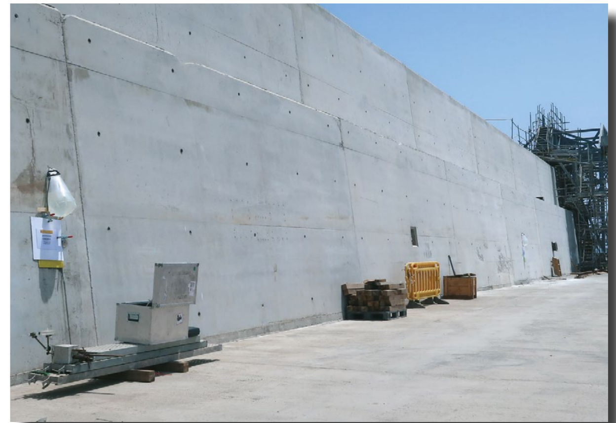
Study of corrosion in the reinforced concrete of the Reina Sofía dock, in the port of Las Palmas.
