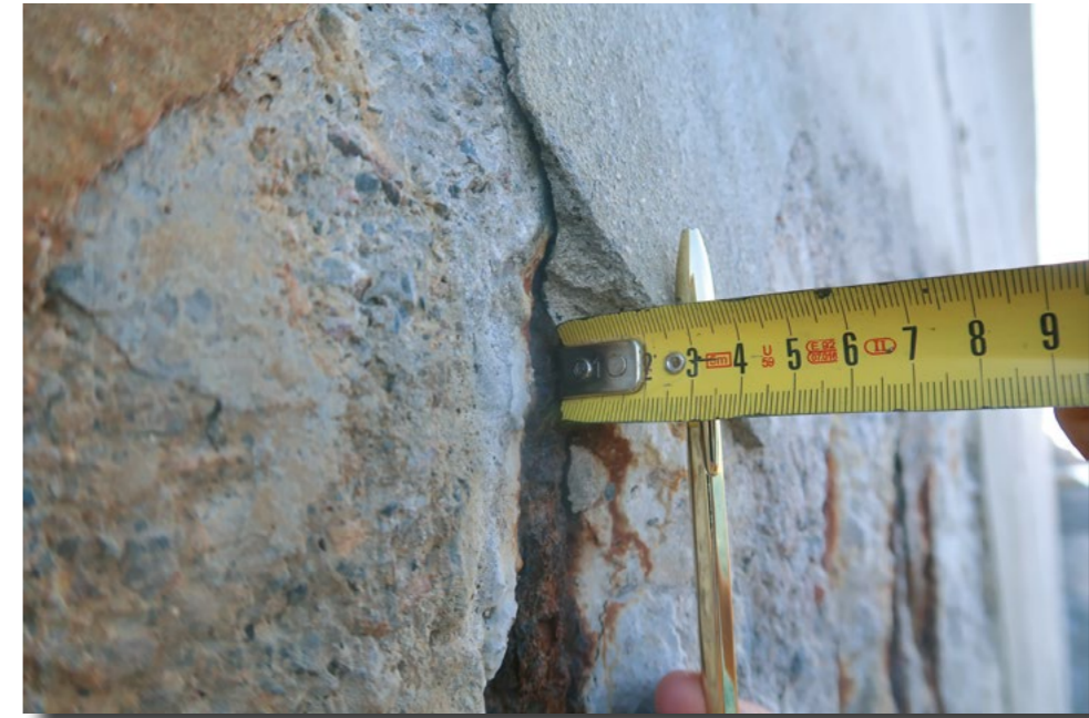
Advanced corrosion due to lack of cover.
